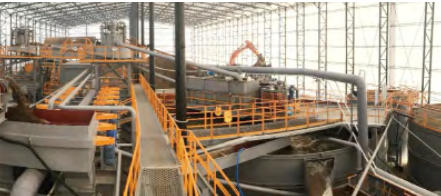
Soil washing facility for complex contamination at Camp Market
